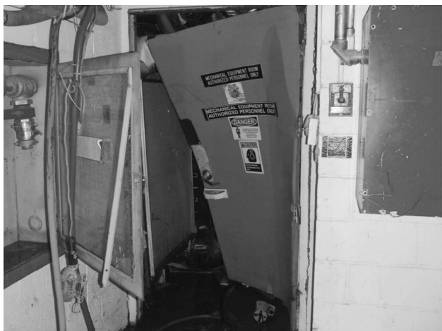
Figure 2 Damage at the NYU Health Sciences Library after Superstorm Sandy
