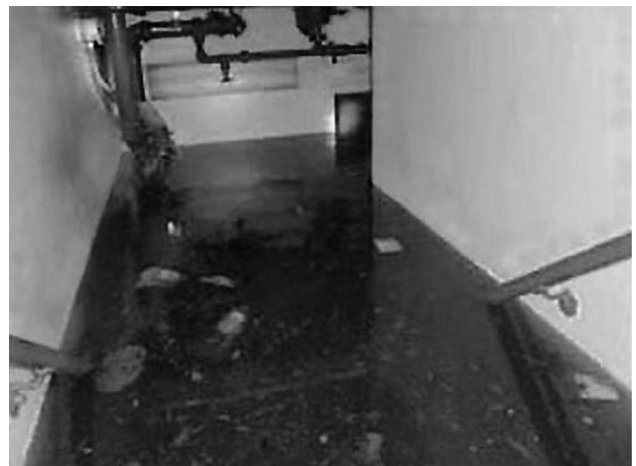
Figure 1 Flooded stairwell of the New York University (NYU) Health Sciences Library after Superstorm Sandy
